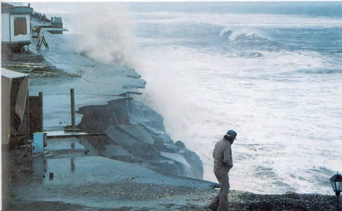
Ocean shorelines are constantly changing, sometimes causing damage to coastal communities. This California roadway was washed away by the pounding of ocean waves.
